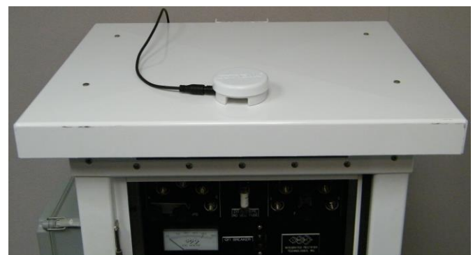
Mounted on rectifier cabinet
