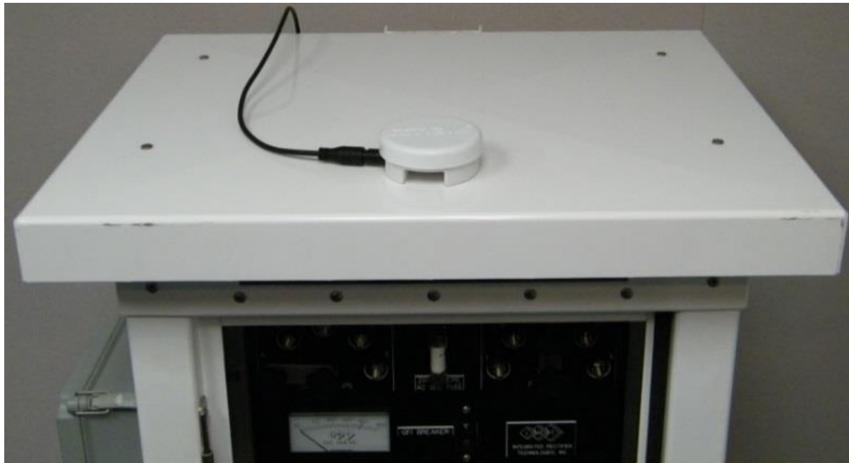
Figure 27 Mounted On Top of a Rectifier Cabinet (uGI1 LCD Display Facing Down)
