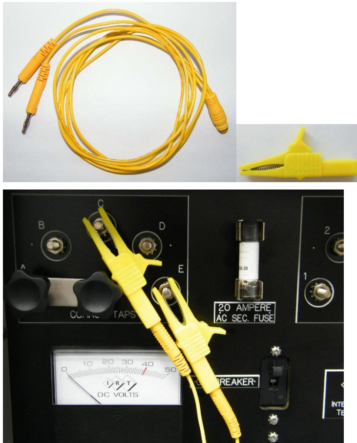
Figure 24 SRL2 Power Cable Clips To Rectifier Taps
