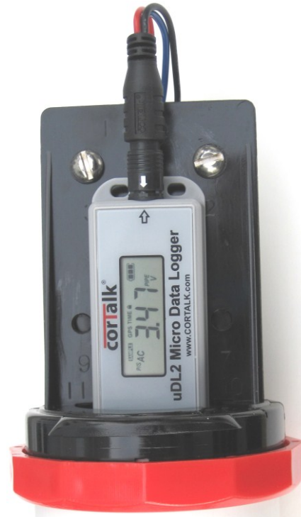
Positioned inside a CP test station
