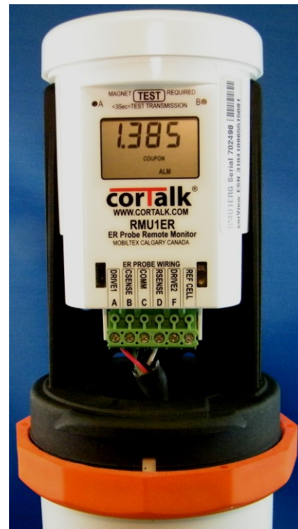
Installed inside a CP test station (cover removed)
