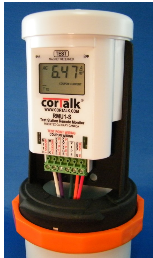
Installed inside a CP test station (cover removed)
